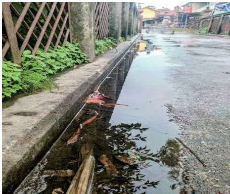
Fig. 5 Water stagnation observed on the deck surface of the Sankhamul Bridge, an old reinforced concrete T-beam bridge.
