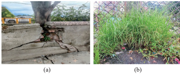
Fig. 4 Deterioration observed in the Sanepa Suspension Bridge (Teku–Sanepa Bridge), a Rana-period suspension bridge constructed in 1940 AD with masonry piers and abutments supporting an early cable suspension system. (a) Tree root growth causing cracking in the masonry elements of the bridge and; (b) grass growth at the base of the parapet, illustrating vegetation-induced deterioration in this historic bridge structure.
