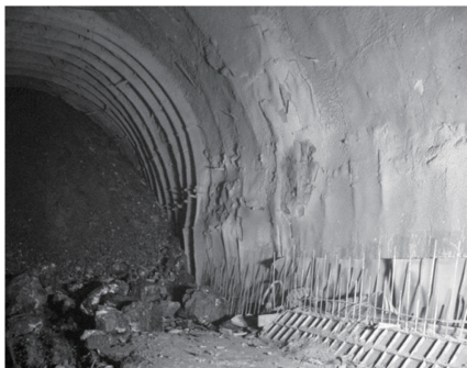
Fig. 1 The initial support of the tunnel is deformed and damaged due to the creep of surrounding rock
