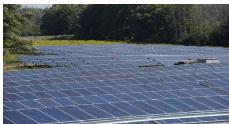
Fig. 5 Solar farm at RIT [41].
